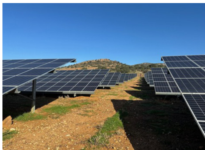
Puertollano II solar park
