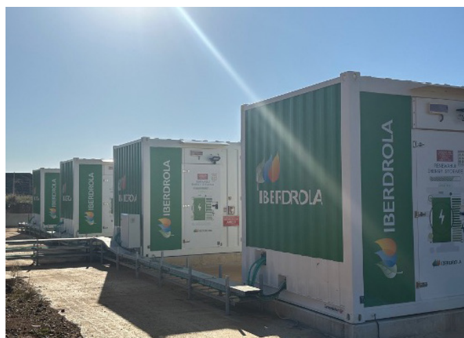
Collocated battery storage
